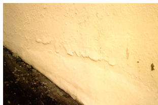
Figure 46. The bubbling of paint shown above is a “balloon” of moisture from the wet masonry surface behind which cannot escape the oil based painted surface
