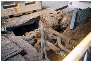
Figure 56. Excavation for footpath works (above) can uncover archaeologically sensitive relics and significant services to adjoining buildings, and needs careful pre-planning.
