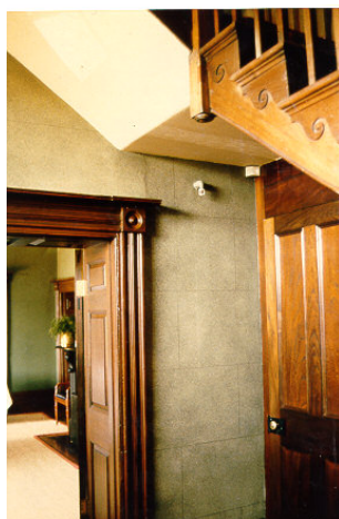
Figure 17. A discreet sprinkler head at Juniper Hall
