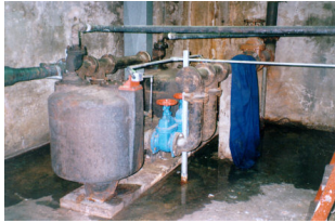
Figure 39. Sewage ejector pots are becoming increasingly rare because they are replaced by many people who consider them antiquated. However, the technology remains sound and if in good condition these pots can usually be retained.
