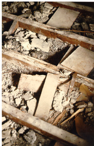
Figure 52. Sand and lime pugging, in this instance between joists, was a common form of sound and thermal insulation
