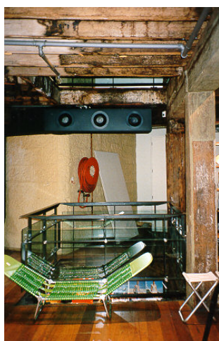
Figure 19. Exposed hose reels in the Argyle Centre, Sydney
