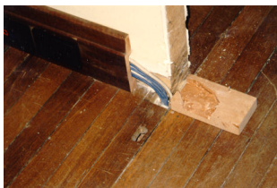
Figure 40. Wires can be easily threaded through floor cavities and behind purpose designed skirtings as above.
