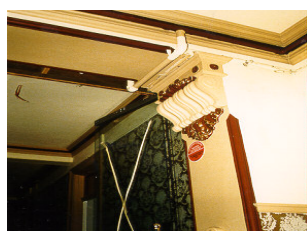
Figure 10. Glass smoke doors at the Carrington Hotel are held open on magnetic catches and close automatically if smoke is detected
