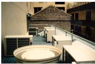
Figure 41. Discreet installation of mechanical plant at roof level
