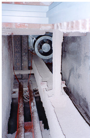
Figure 27. This services stack, housing essential services (under construction), is located in a former air shaft and light well area which was infilled during the mid 20 th century
