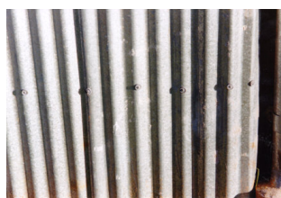
Figure 43. Something as simple as roof fixings will have an impact on the significance of a place if not undertaken in a proper, traditional manner. Domed slotted screws with lead washers can still be sourced if the desire is there
