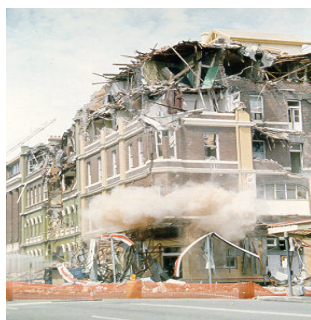
Figure 4. This building in Newcastle, supposedly in danger of imminent collapse, took a ball and chain crew nearly all day to demolish.
