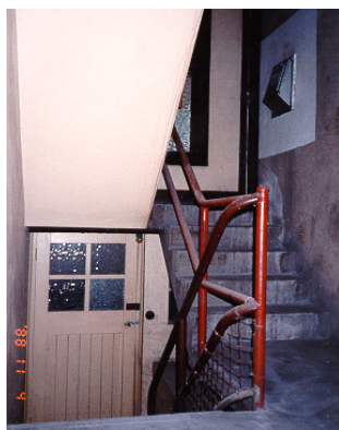
Figure 11. Existing service stairs in an Inter-War block of flats, Potts Point, Sydney
