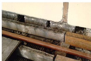
Figure 21. Sprinkler pipes were concealed within the floor space of this traditional building during repairs to joists and floorboards, allowing other fabric to remain undisturbed.
