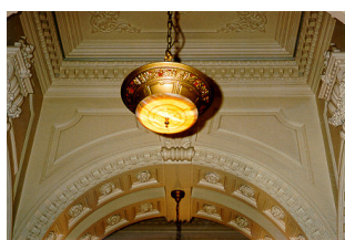
Figure 22. Existing light fittings in Sydney Town Hall also serve as emergency lights.
