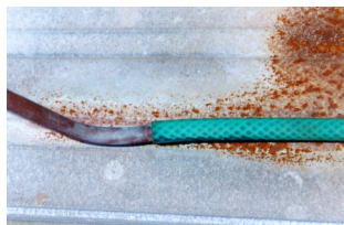
Figure 42. Where incompatible metals are in contact, or water flows from one to another, rapid corrosion may occur. In this example, a copper condensate drain has corroded the galvanised steel tray and been extended in a crude manner with ordinary garden hose.
