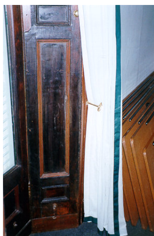
Figure 16. These 1830s cedar joinery elements survived a fire with protection from their original shellac covering.
