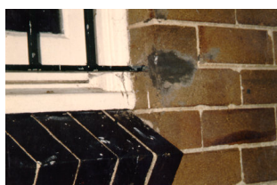
Figure 47. Poorly prepared and maintained ferrous fixing in this instance has caused breakdown in the masonry reveal. Note the inappropriate patching in hard cement based mortar
