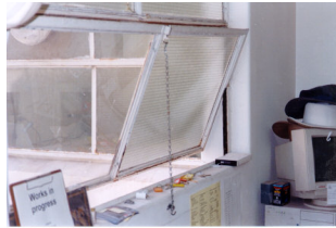
Figure 50. Wired glass fire resistant window as shown in the original pane below
