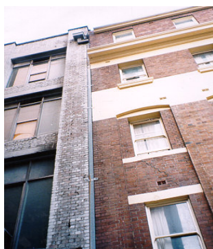
Figure 2. This crack looks serious, but has existed for many years without change and is not affecting structural stability
