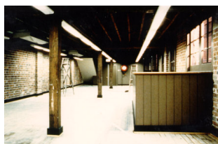
Figure 48. The hardwood framing conserved in this warehouse was previously exposed to fire, with minimal charring of the structural members.
