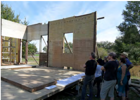
Re-erection of a prefabricated timber cottage International Day of Monuments and Sites at Gulf Station (Natica Schmeder)
